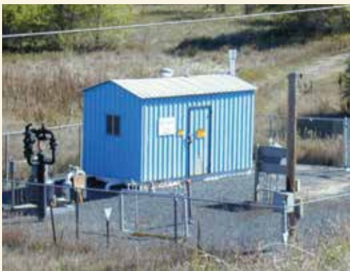
City gate meter station.
