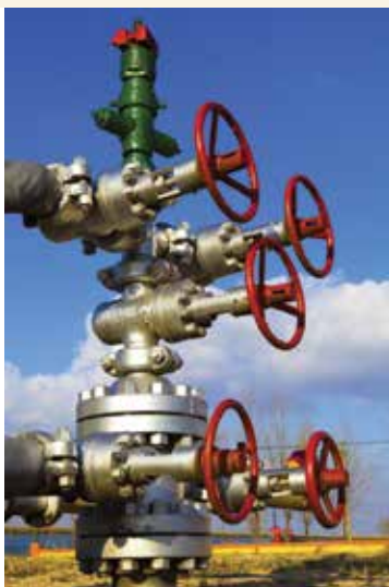
Natural gas wellhead.
