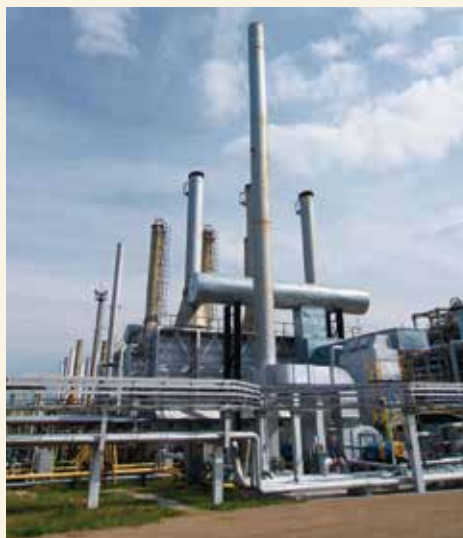
Natural gas processing facility.
