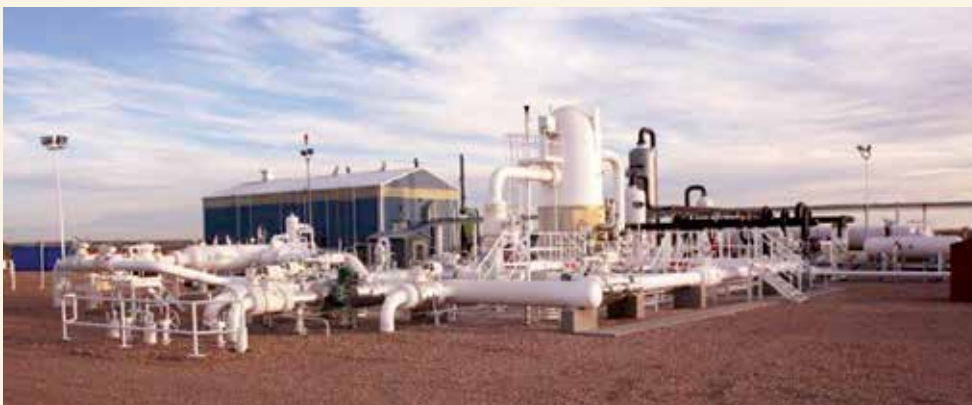
Natural gas compressor station.
