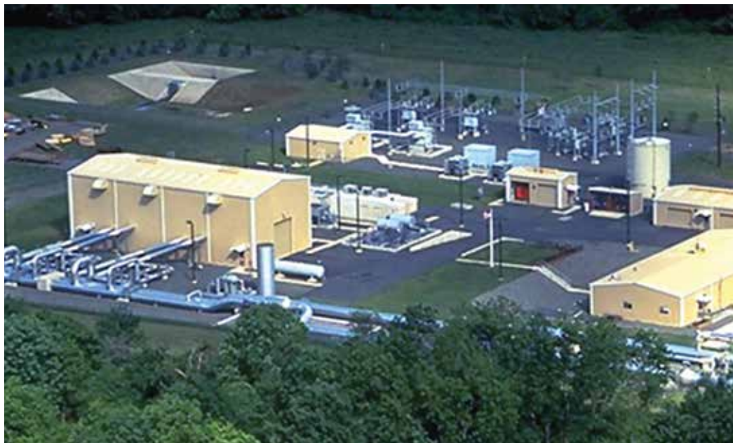
Gas transmission compressor station.
